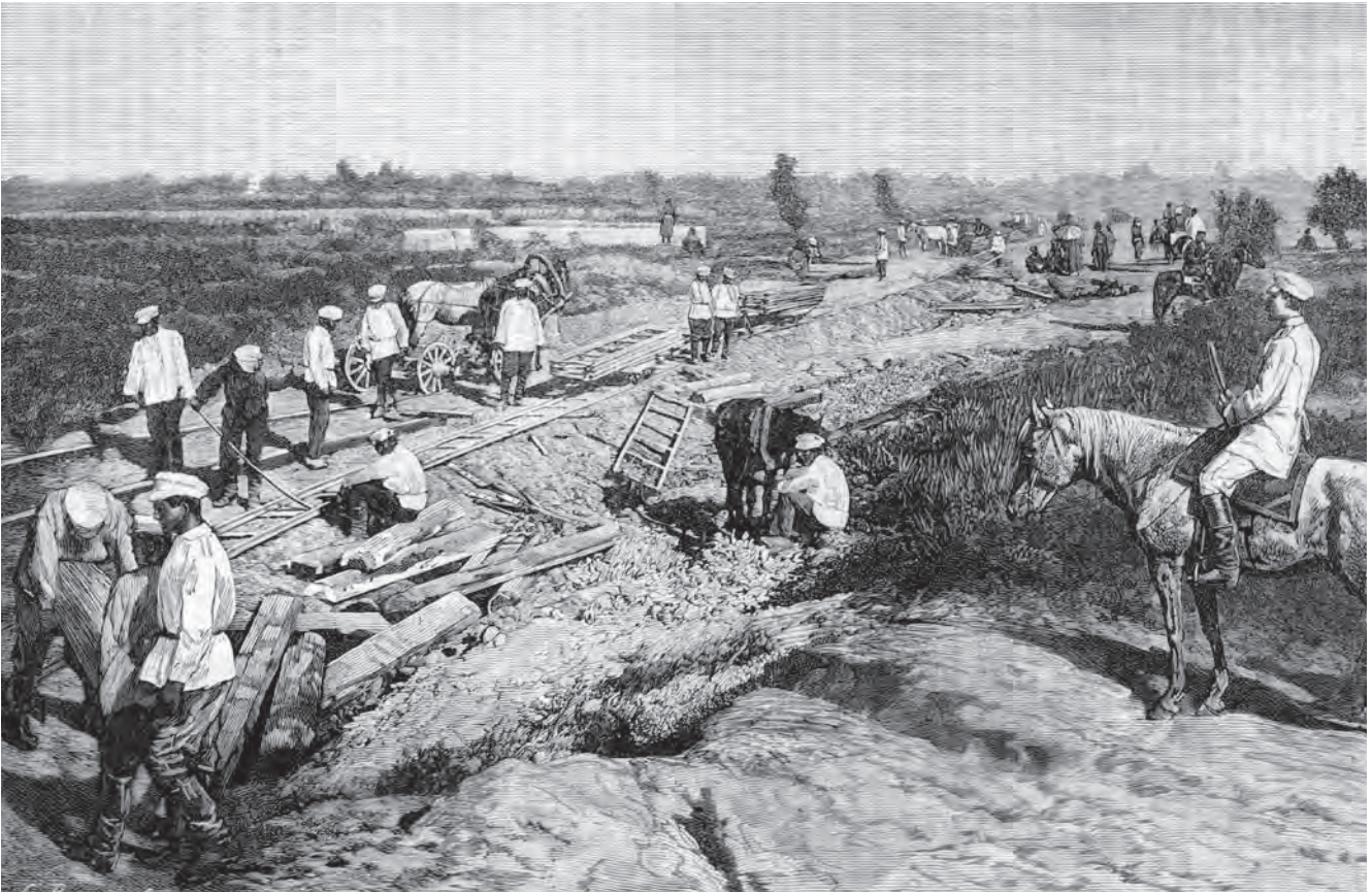
Pictured: Construction of the trans-Caspian Railway. Photo: Universal History Archive/Universal Images Group via Getty Images
